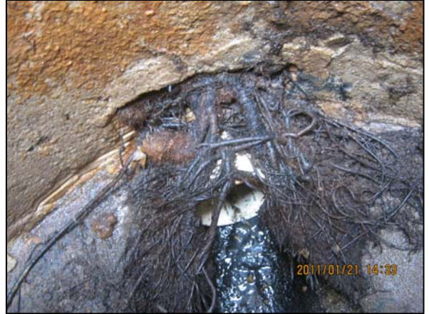
Cracked Pipe Seal with Roots (RV14)2846
