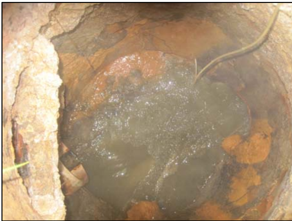
Deteriorated Manhole (RV07)1001
