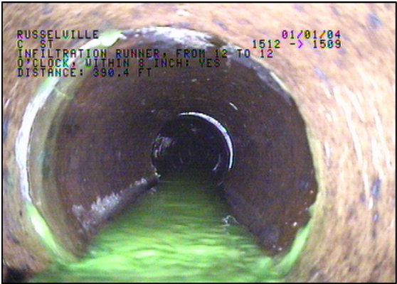
Separated Joint with Infiltration (RV23)1512-1509
