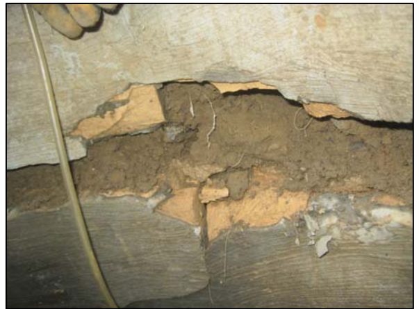
Broken Corbel (RV07)1829
