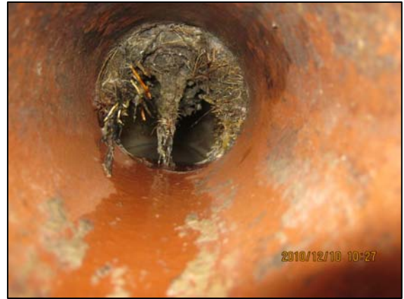
Roots at Joint (RV07)6106
